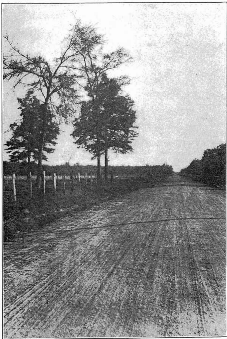
Fine gravel roads are to be found in many parts of Arkansas. The road shown above, Federal Aid Project No. 98, Road Improvement District No. 12, Woodruff County, is typical of the many miles of roads of this character built during the past several years.
